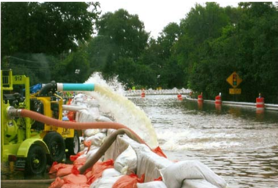
September 2008 Flooding of Des Plaines River at River Road
