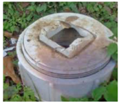
Improperly capped cleanout
