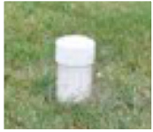
Properly capped cleanout
