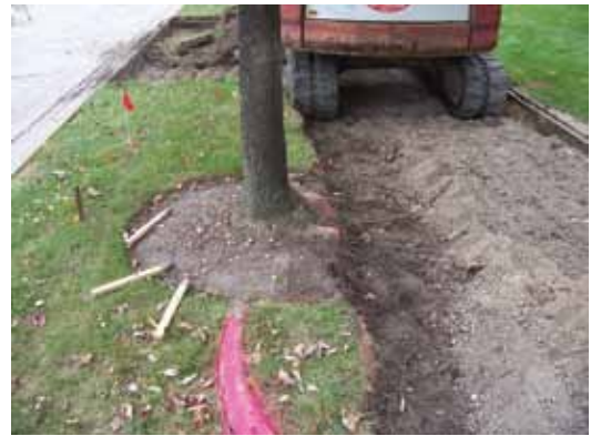
Photograph 3G-4. Tree root damage as a result of construction activities on Pine St.
