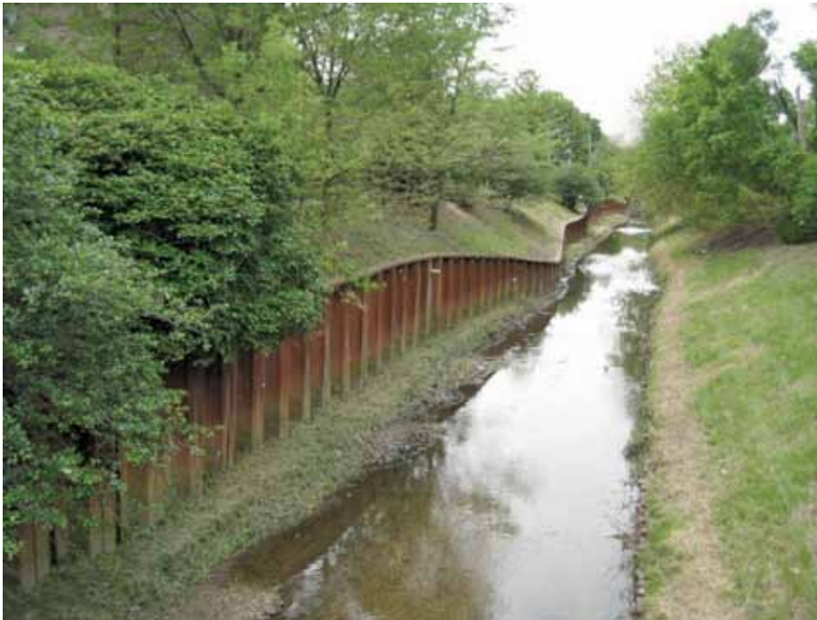
Photograph 3Q-1. A well maintained section of Weller creek where bank stabilization has been installed. Creek and drainage maintenance is important to keep trees and branches from blocking drainage, stabilizing creek banks and protecting property flooding and erosion, and to eliminate breeding locations for pests.
