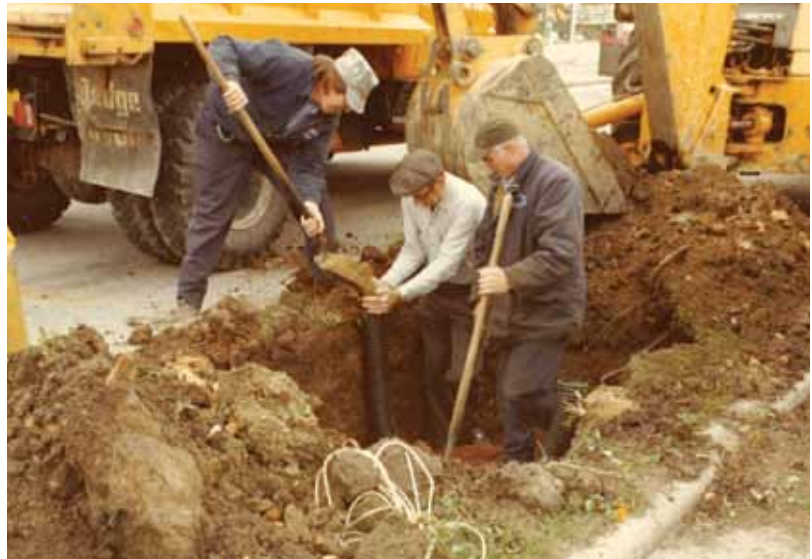
Photograph 3D-2. A drainage sump being installed in a tree planting site in May 1975 in the Village to modify the site and make it more amenable to planting.
