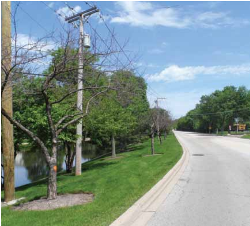
Photograph 2C-1. The drought of 2012 directly killed many trees such as these in the Village. Experts predict that periods of drought are likely to become more frequent in the future as a result of climate change.
