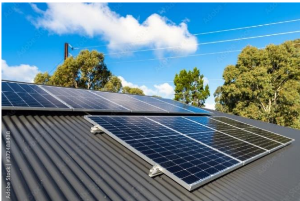
Rooftop Solar Panel
