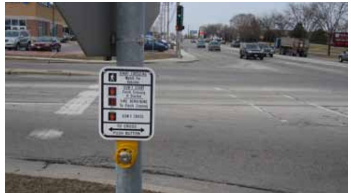
Figure 33: Example of an actuated crosswalk signal
