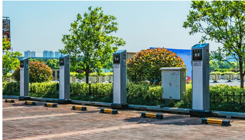
Electric vehicle charging stations.
