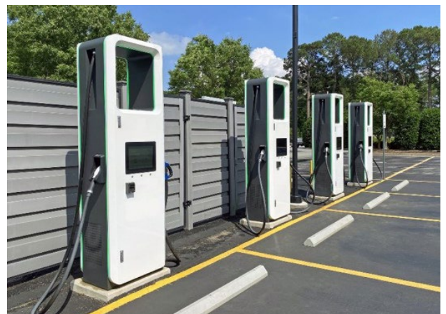
Electric Vehicle Charging Stations
