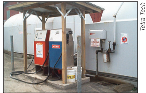
Figure 8. Spill kits should be maintained in areas with spill potential, such as fueling stations.
